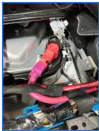
DC-DC "penthouse" lug under rear seat (~15-15.5VDC)
