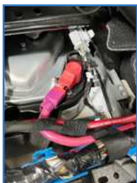
DC-DC "penthouse" lug under rear seat (~15-15.5VDC)
